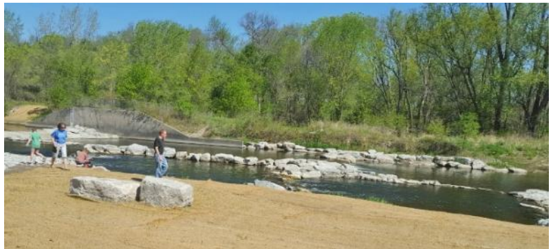
On left, Steve and Teri Veysey representing HFFA at ribbon cutting ceremony Finished project ,above
